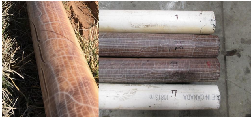
Figure 1: UV Cracking Damage to Surface Pipeline
