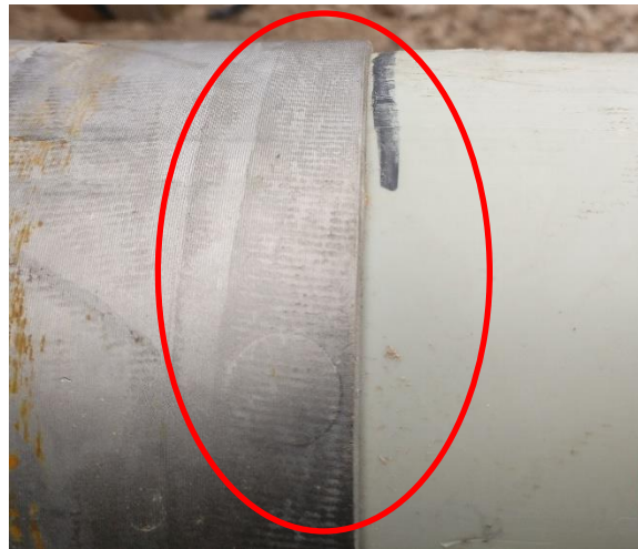
Figure 244: No Visible Flare
