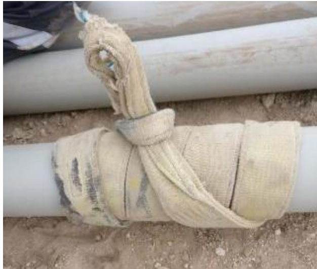
Figure 93: Sling Wrap on Pipe
