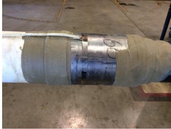
Figure 250: Anode Fixed to Fitting Sleeve
