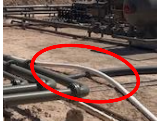
Figure 158: Unacceptable Unsupported Line Crossing
