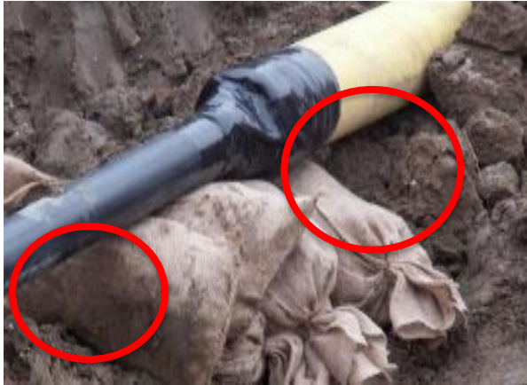
Figure 146: Insufficient Sandbag Support
