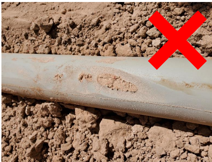
Figure 156: Pipe Damage from Abrasion Against a Solid Surface
