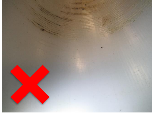
Figure 238: Poor O-ring Seal
