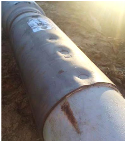
Figure 243: Improper Die Bolt Impressions
