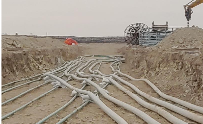
Figure 159: Multiple FlexPipe Lines Crossings Protected by Sandbags
