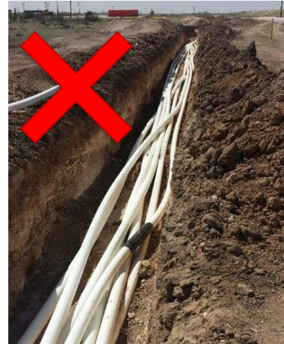
Figure 126: Lines Laid Incorrectly Across Each Other
