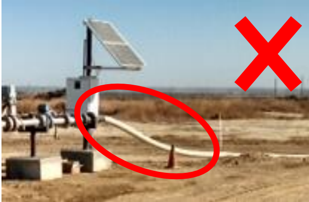
Figure 157: Unacceptable Unsupported FlexPipe on Surface
