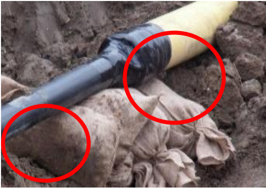
Figure 8: Insufficient Sandbag Support
