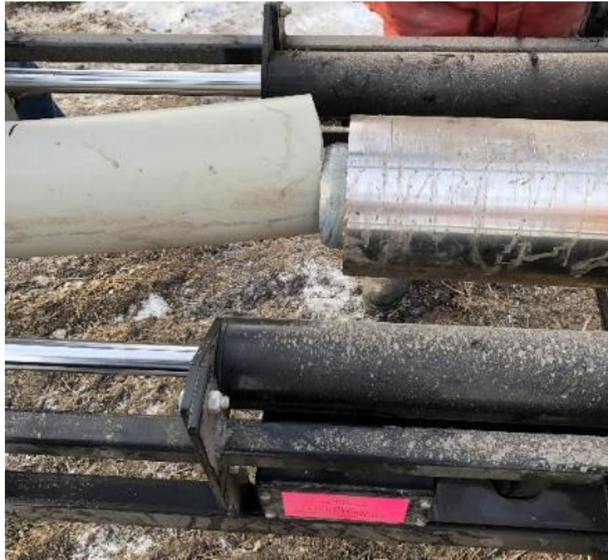
Figure 30: Misaligned pipe and fitting
