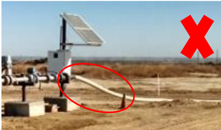
Figure 5: Unacceptable - above ground connection must be at a 45-degree angle for surface pipelines
