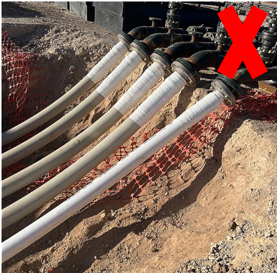
Figure 4: Improperly supported virgin soil riser - pipeline is not supported by virgin or compacted soil
