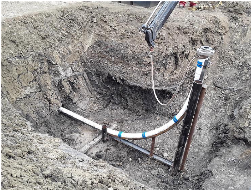
Figure 1: Flexpipe installed in a Flexpipe riser chute
