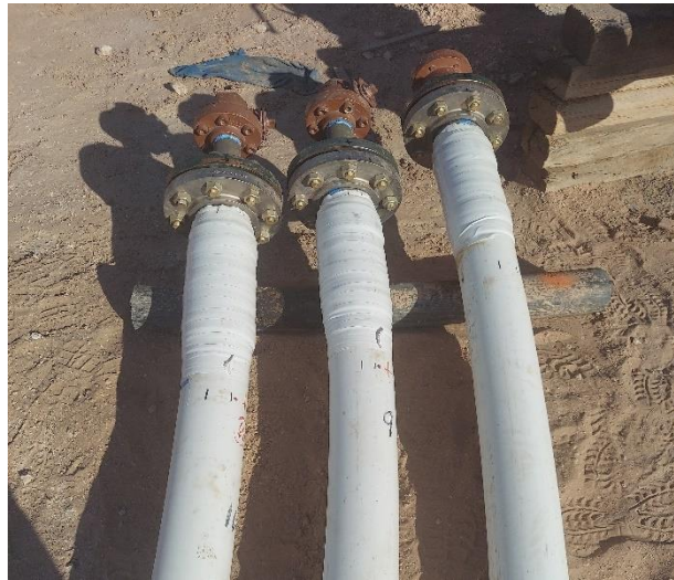
Figure 14: Allow at Least One End of the Pipeline to Rotate Freely During the Pressure Test
