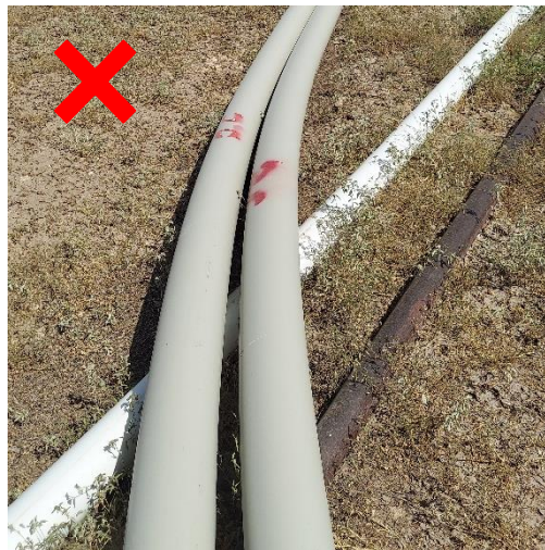
Figure 8: Unacceptable Unsupported Line Crossings
