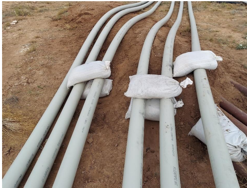
Figure 18: Separating Pipe Crossings with Protective Material such as Sandbags or Sand Piles
