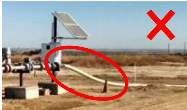
Figure 4: Unacceptable Above Ground Connection - Surface Pipeline Connections Must be at a 45-Degree Angle
