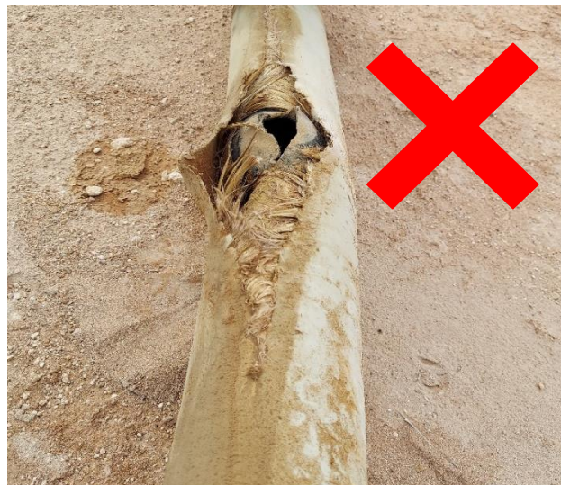
Figure 6: Pipe Damage from Abrasion Against a Solid Surface
