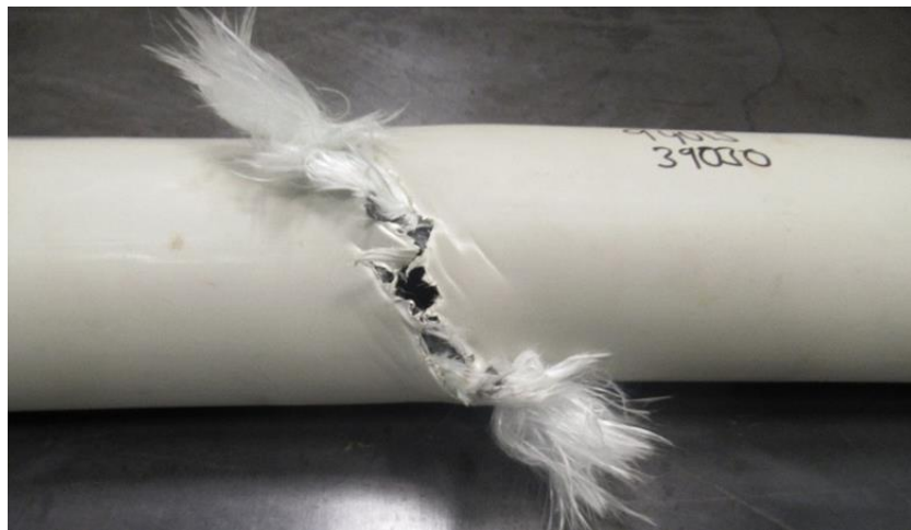
Figure 1. Example of a burst pipe damage
