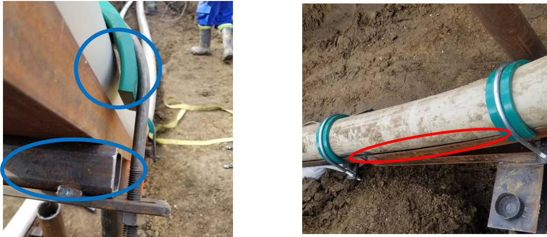
Figure 16: Square backing tubing and gap between the plastic half-moon and the pipe (left). Gap between the pipe and C-channel (right).
